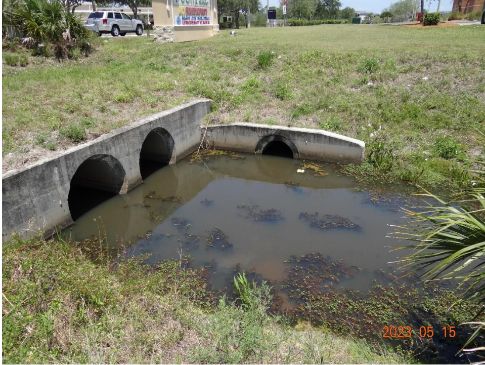
POND A OUTFALL PIPE
